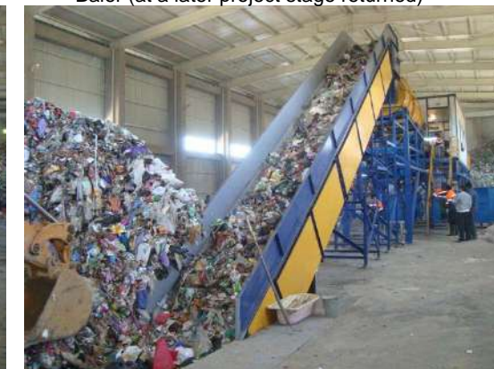
Waste feeder in operation
